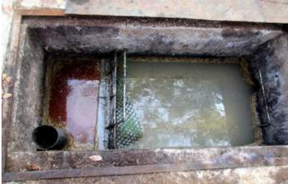
Figure 4.3 Tank for removing sediments and floating matter from canteen waste water before reaching ETP
