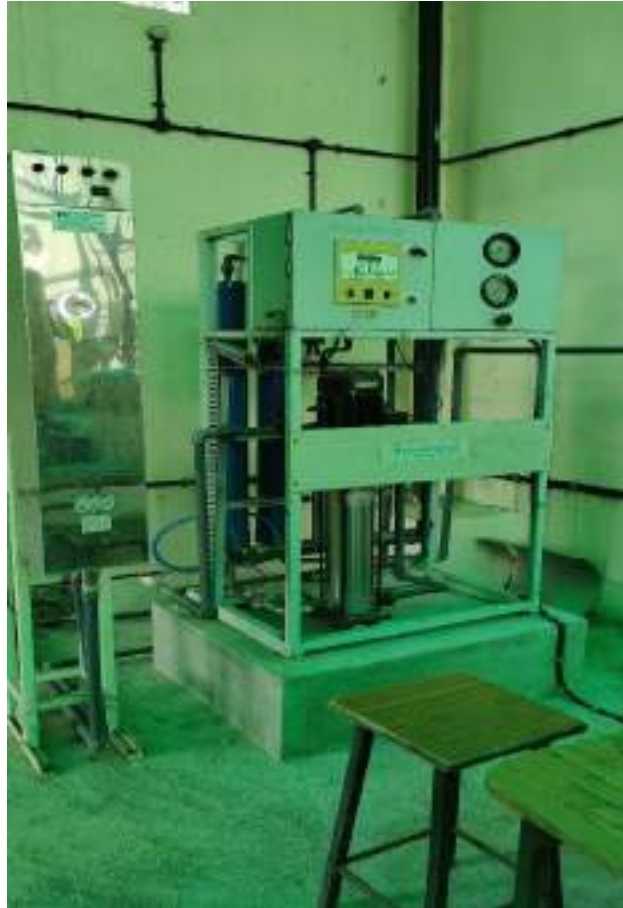
Figure 2.8 Reverse Osmosis unit in ETP of SSET campus
