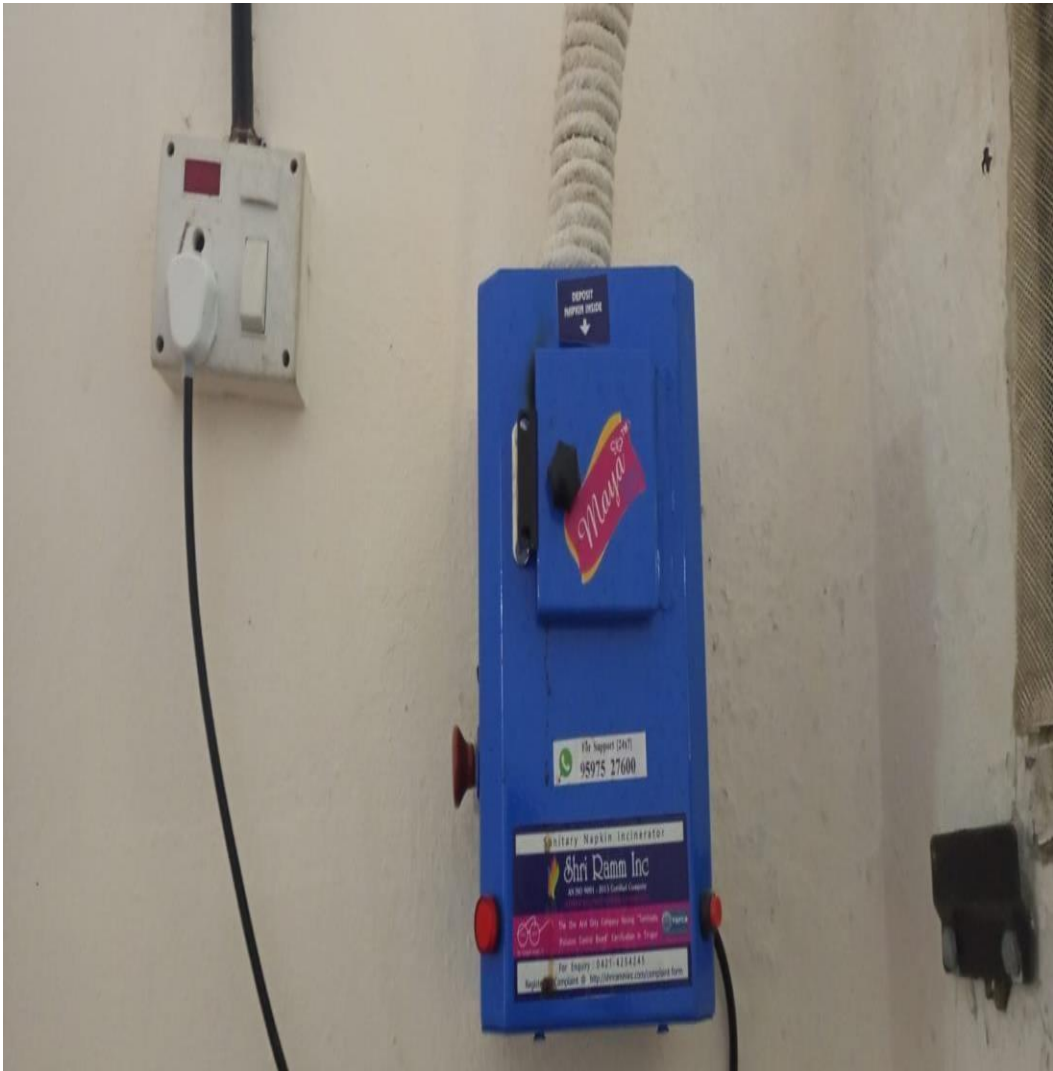
Electrical Sanitary pad Incinerator
