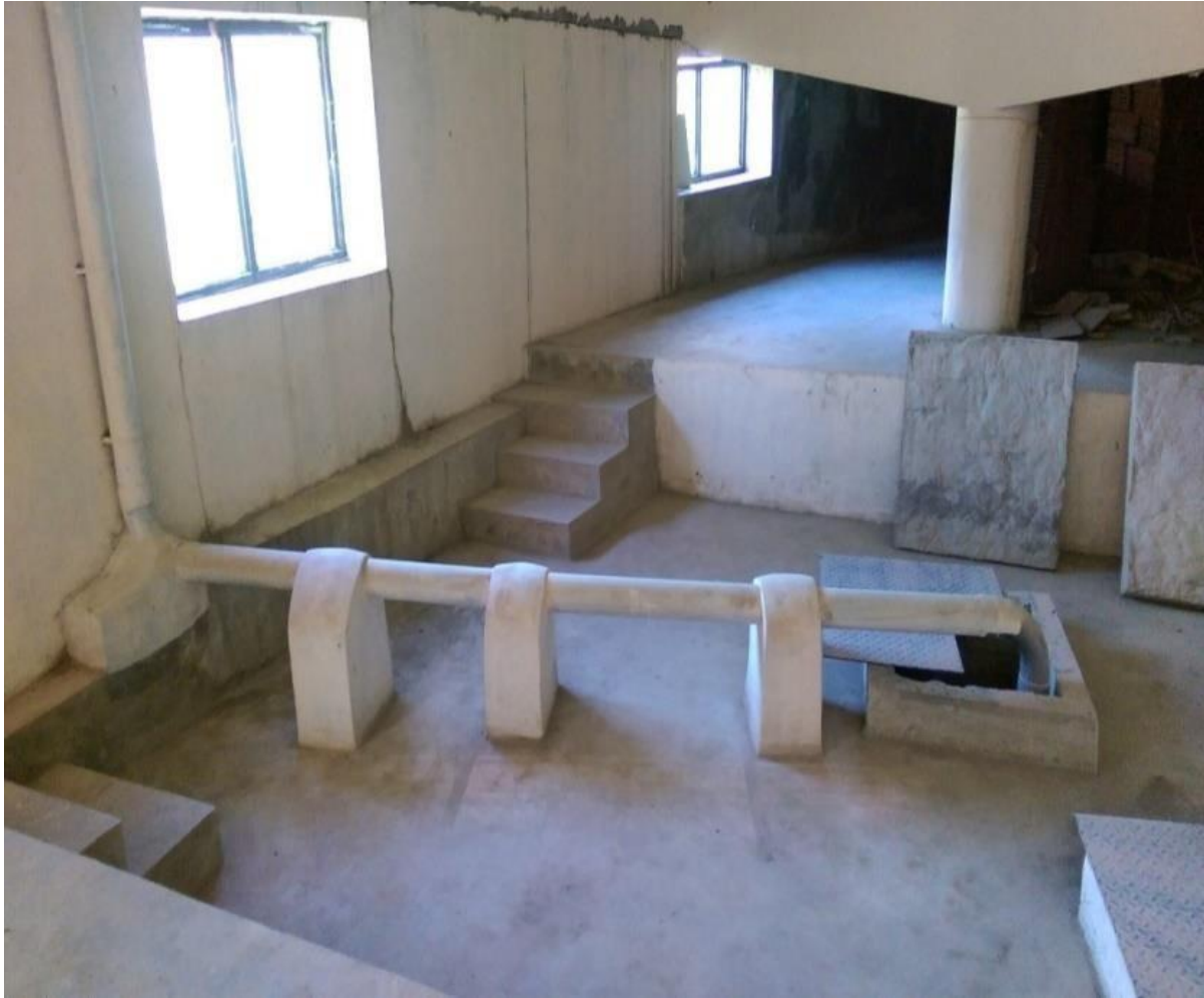
Fig. 2.11 Rain water collected at rooftop directed open well for recharging
