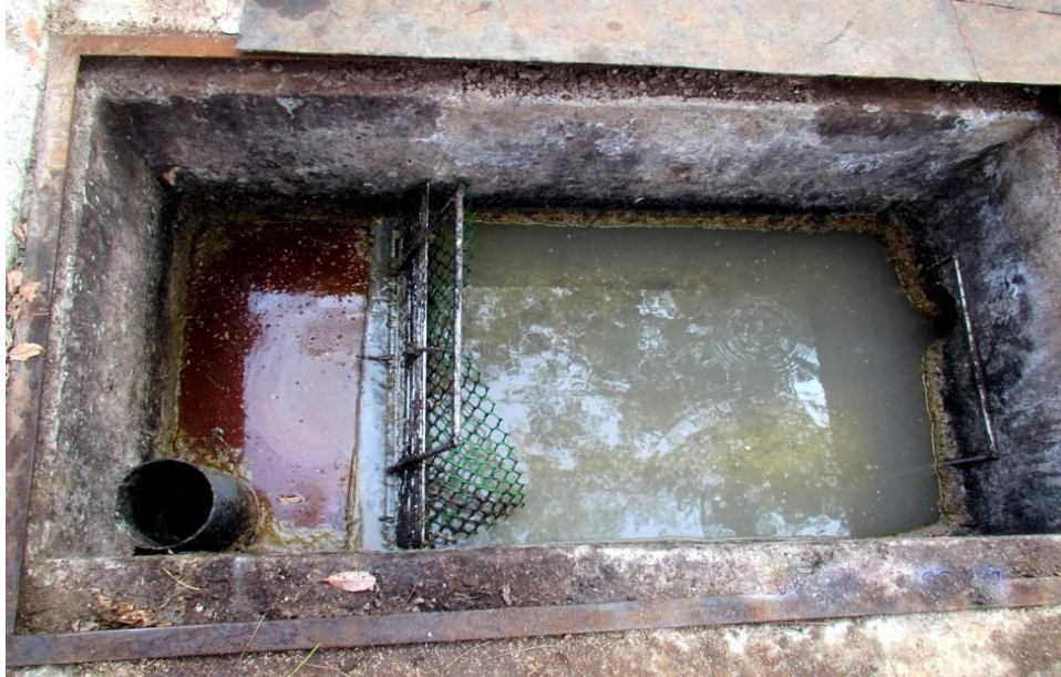
Figure 4.3 Tank for removing sediments and floating matter from canteen waste water before reaching ETP
