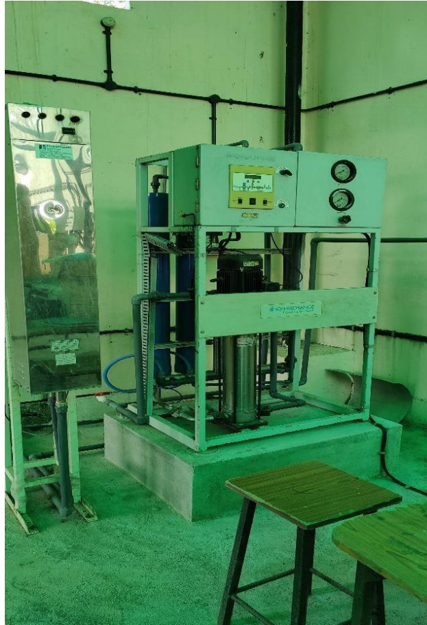
Figure 2.6 Reverse Osmosis unit in ETP of SSET campus
