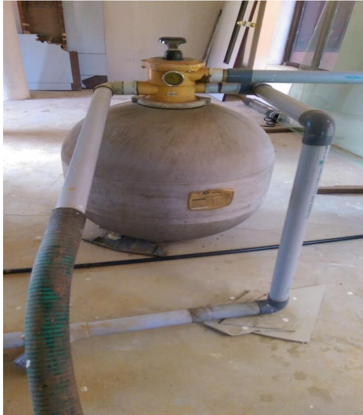
Figure 2.9 Rain water collected at rooftop is treated using Pressure sand filter before taken for bore well recharge
