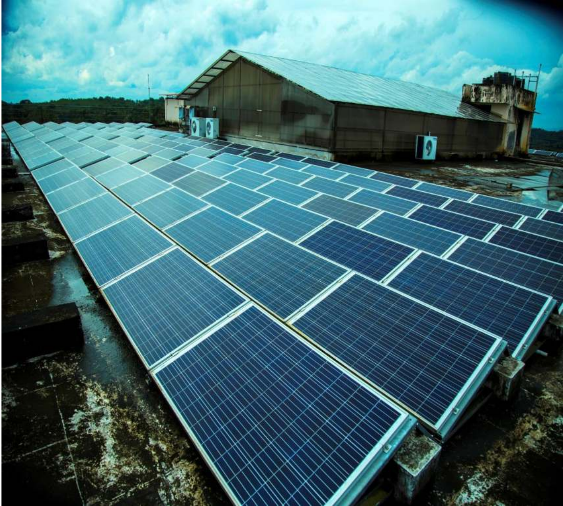
Roof Top Solar Power System
