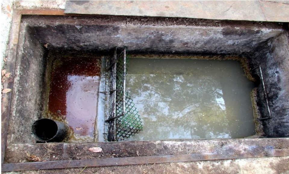
Figure 1.6 Tank for removing sediments and floating matter from canteen waste water before reaching ETP
