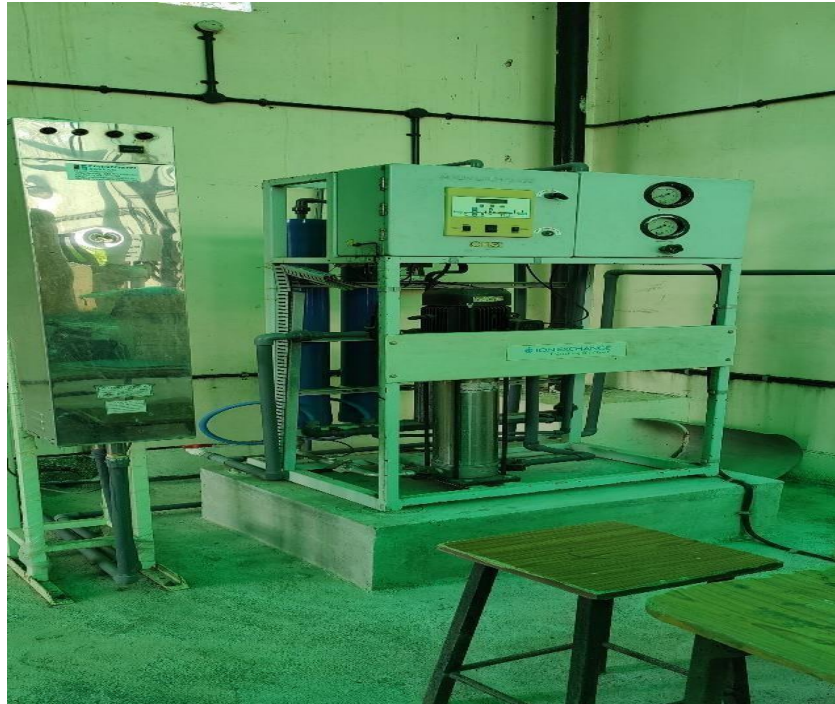
Figure 1.2 Reverse Osmosis unit in ETP of SSET campus
