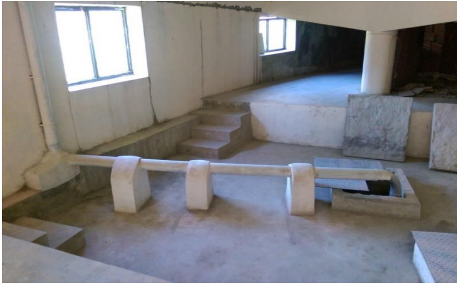
Fig.3. Recharge well. Rainwater collected from rooftop after filtration is recharged into an open well
