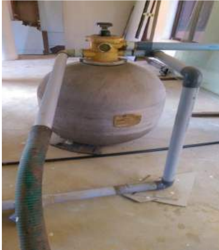
Figure 2.12 Rain water collected at rooftop is treated using Pressure sand filter before taken for bore well recharge
