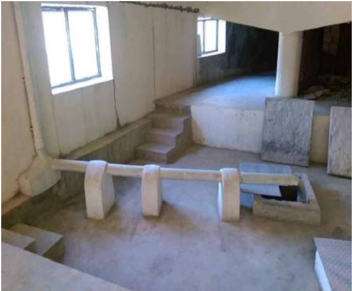
Fig. 2.14 Rain water collected at rooftop directed open well for recharging
