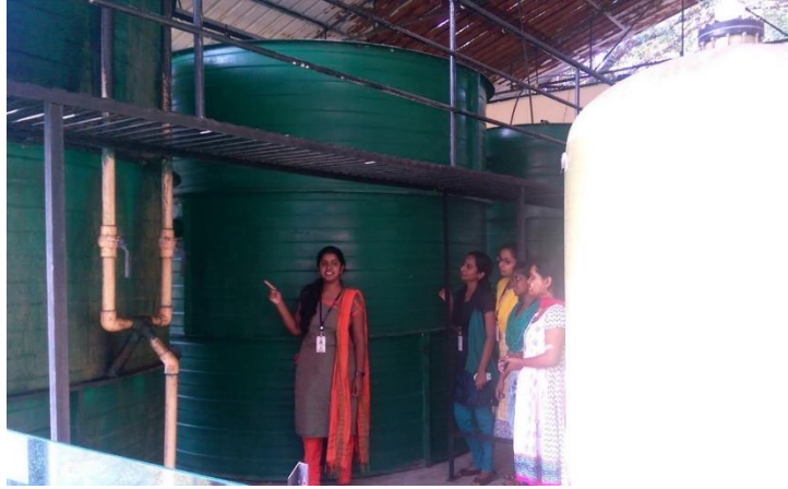
Fig.7 Aerobic MBBR tanks at STP
