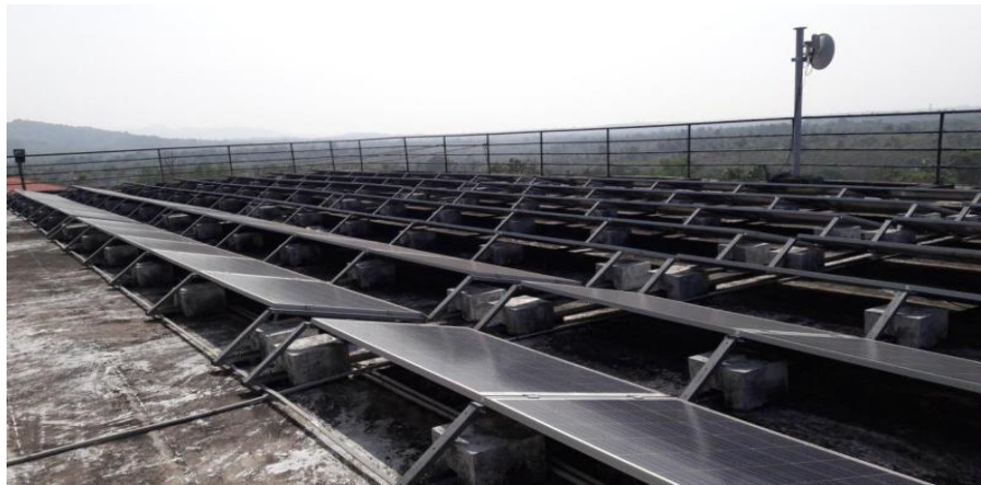
Fig. 5 Solar panels of 50 KWp ON-GRID solar power plant at SSET
