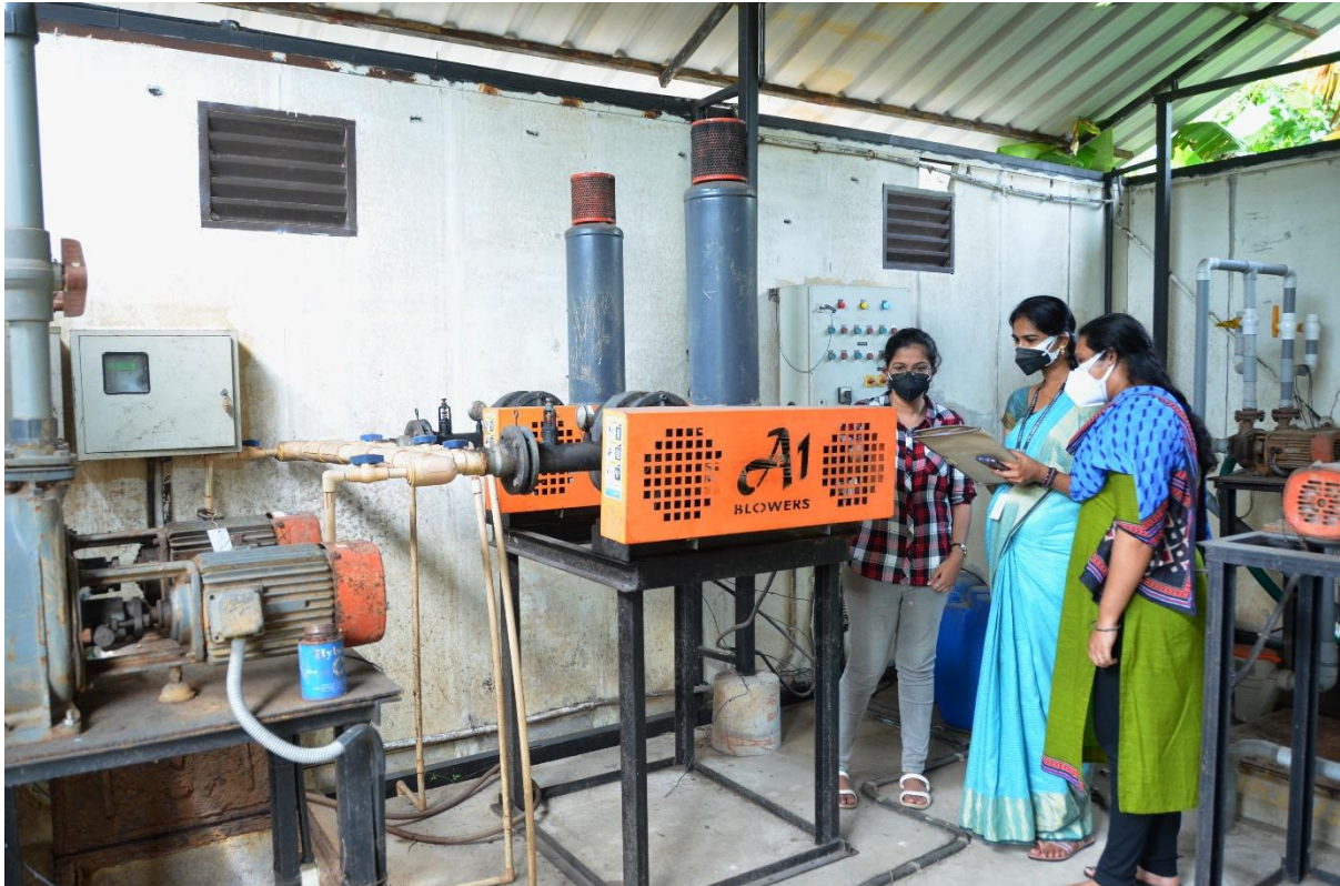
Fig 2.4 The audit team examining sewage treatment plant
