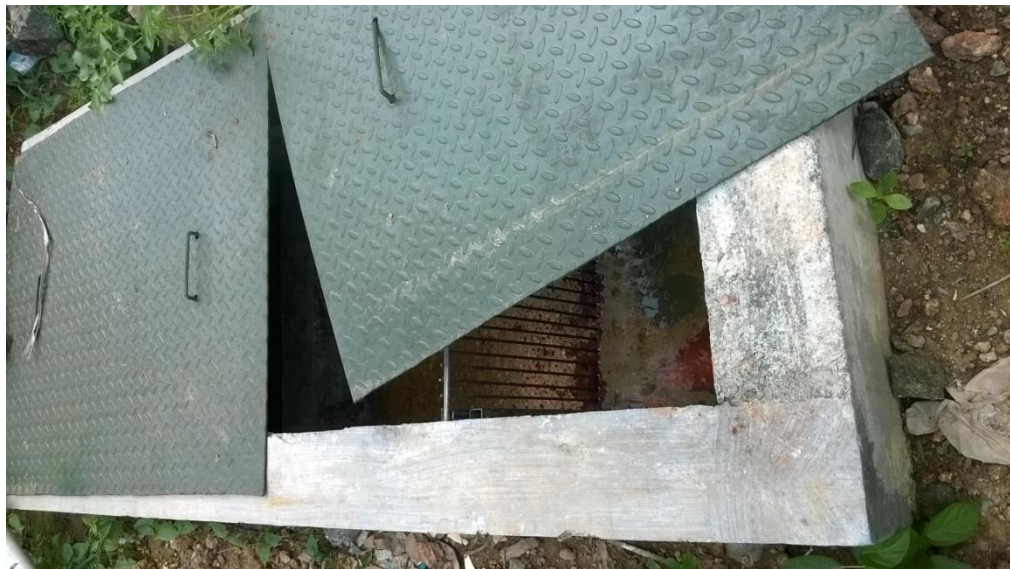
Figure 4.4. Tank outside canteen for removing sediments before water is taken to ETP
